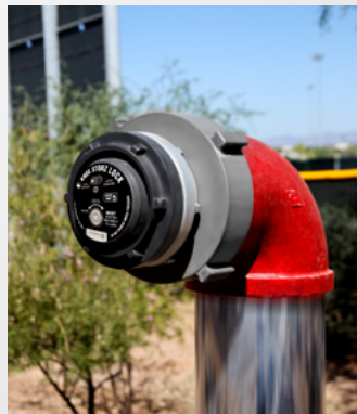
Knox Storz Lock secured onto a large FDC
